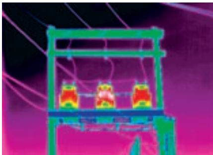
Figure 5-40. A transformer that appears to be operating warmer than others on an elevated rack can be the sign of a potential problem.
