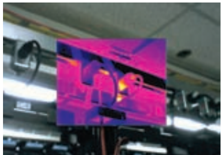
Figure 5-81. The right-hand electrical plug for a bank of computer servers shows a thermal pattern that indicates either a high-resistance connection or an internal wiring problem.
