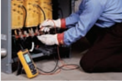
Figure 10-2. Electrical analysis uses electrical monitoring equipment to evaluate the quality of power delivered to equipment.
