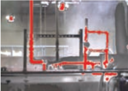
Figure 5-22. The use of saturation colors and color alarms in a grayscale palette can be useful for determining the hot water and steam valves that are open and operating properly.
