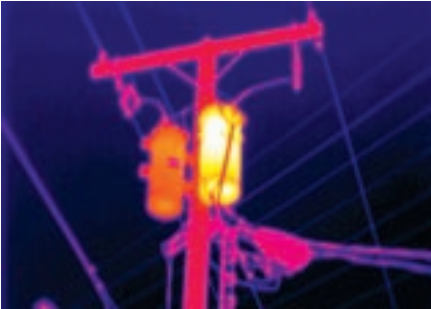
Figure 5-84. This thermal image indicates that the transformer on the right may have an internal fault.
