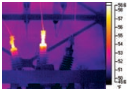
Figure 5-59. Two of the six bushing caps on an oil-filled circuit breaker are abnormally hot and represent a condition that would have proved costly had it not been detected and repaired.
