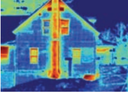
Figure 5-48. A thermal image of the exterior view of a building can clearly show problem areas such as the lighter sections where insulation is missing.
