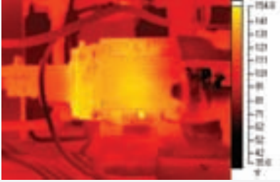
Figure 7-2. Many differences in the thermal signature of the motor will show up in subsequent thermal inspections.
