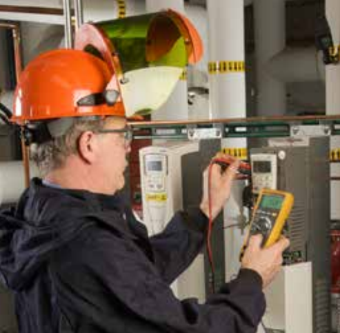
Jim Murphy, Electrical Foreman uses the Fluke 179 DMM to look at low voltage signals in the newly installed VFD for the 40+ year old steam system.
