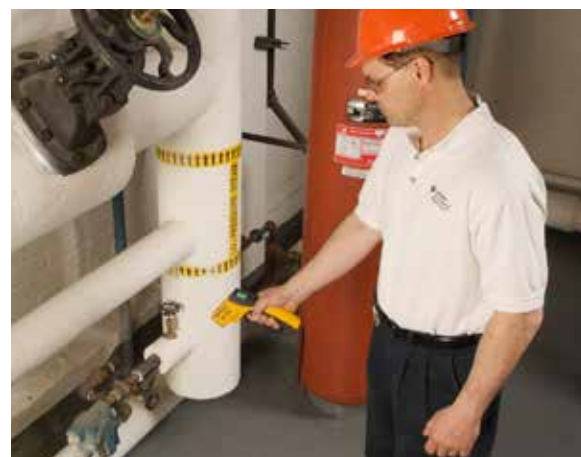
Darryl Dylla, HVAC/Power Plant Manager, uses a Fluke 62 Infrared Thermometer to check steam traps through-out the HVAC system.
