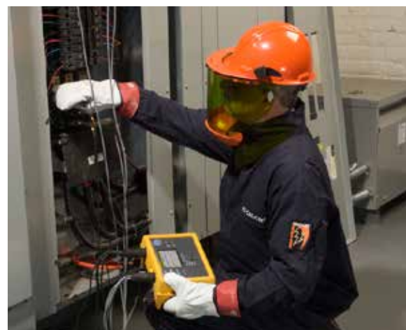
Rolf Zoeller, Electrician uses the Fluke 1735 Three-Phase Power Logger to do load studies on the hospital's electrical systems. Keeping close tabs on these systems helped the hospital achieve its ENERGY STAR rating.
